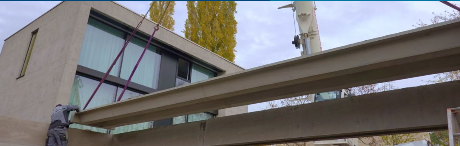
Installation of a trapezoidal slab made of prestressed carbon concrete for a garage
