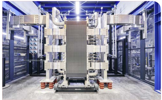
In the H 2 Giga DERIEL project, electrolyser modules are being built on a real scale of one megawatt in test stands.
