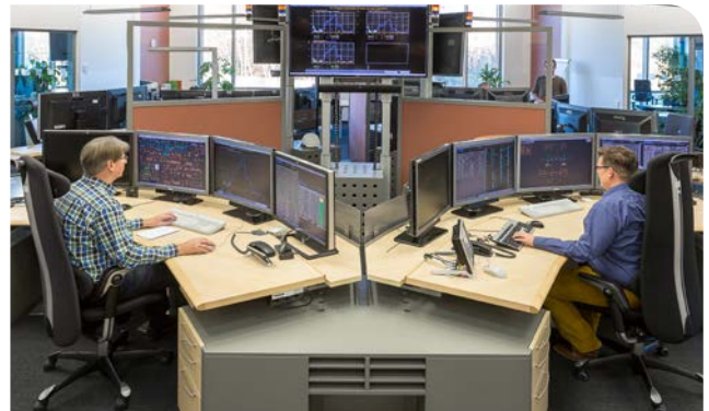
The control centre staff processes information for the electricity and gas supply.
