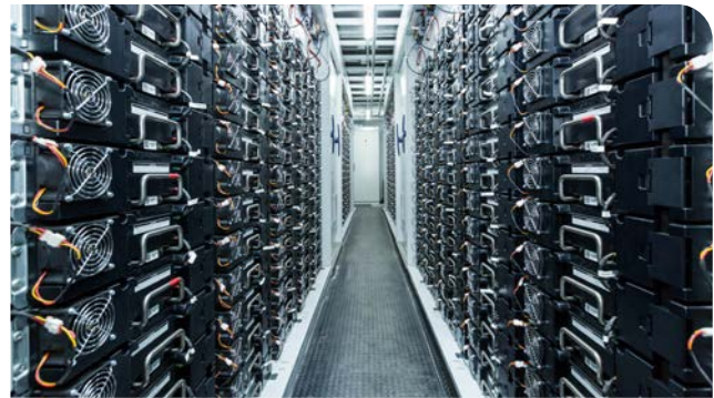
The battery storage system helps to optimise the operation of the Bremen-Hastedt hybrid power plant.
