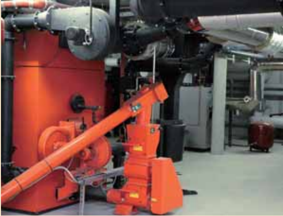
Wildpoldsried village heating system with wood pellets.
