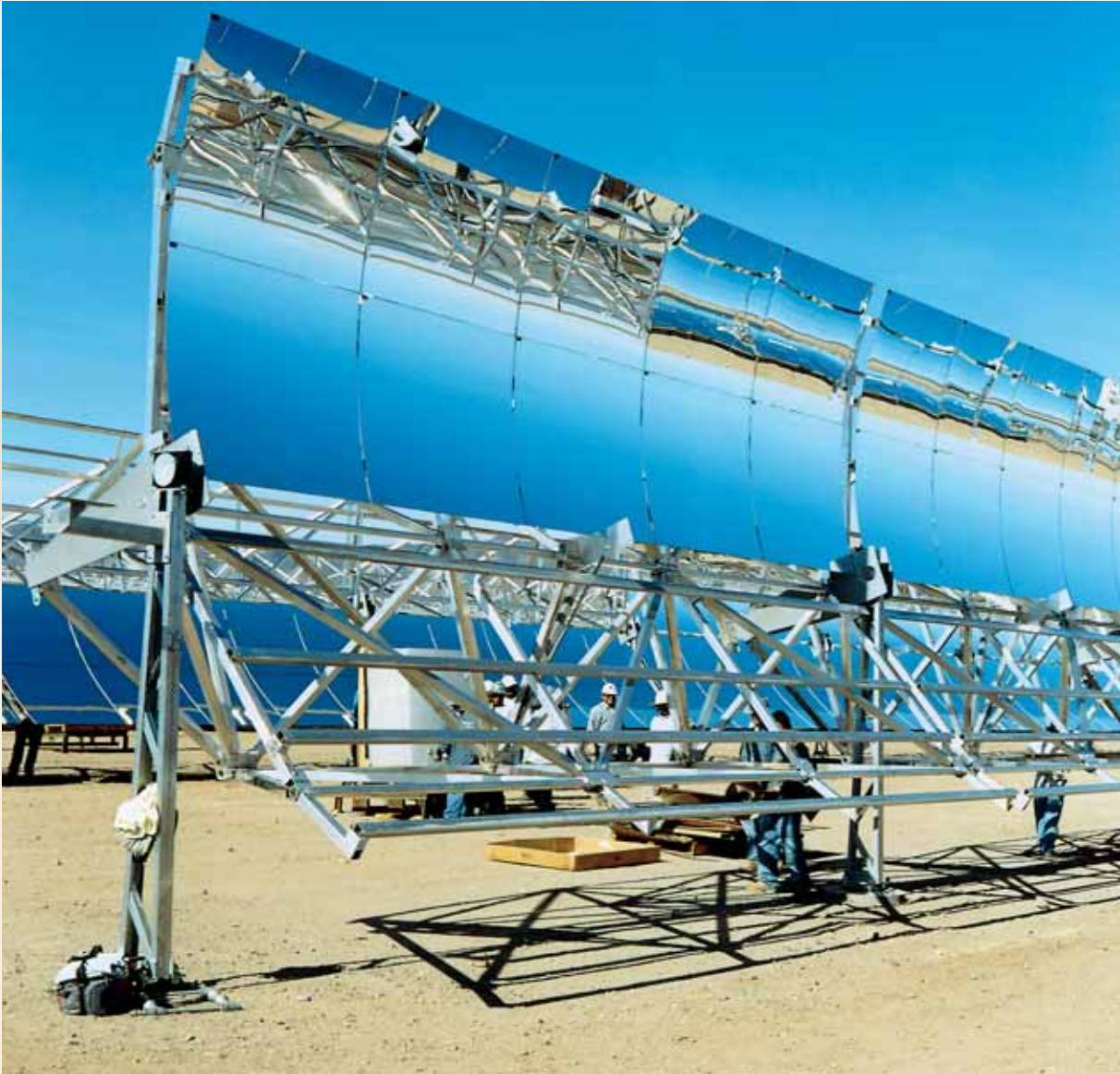
Solar parabolic trough power plant for high-yield sunshine regions.
