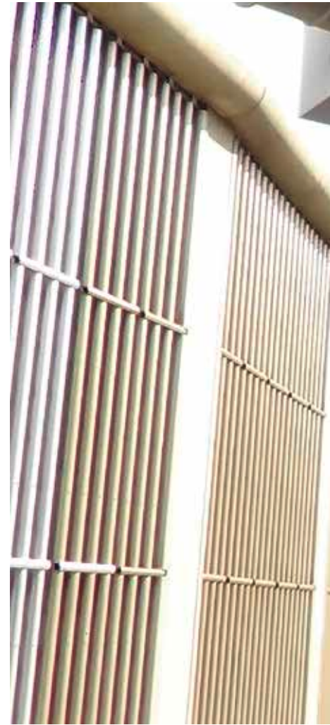
PCC pilot plant for CO 2 scrubbing in Niederaußem
