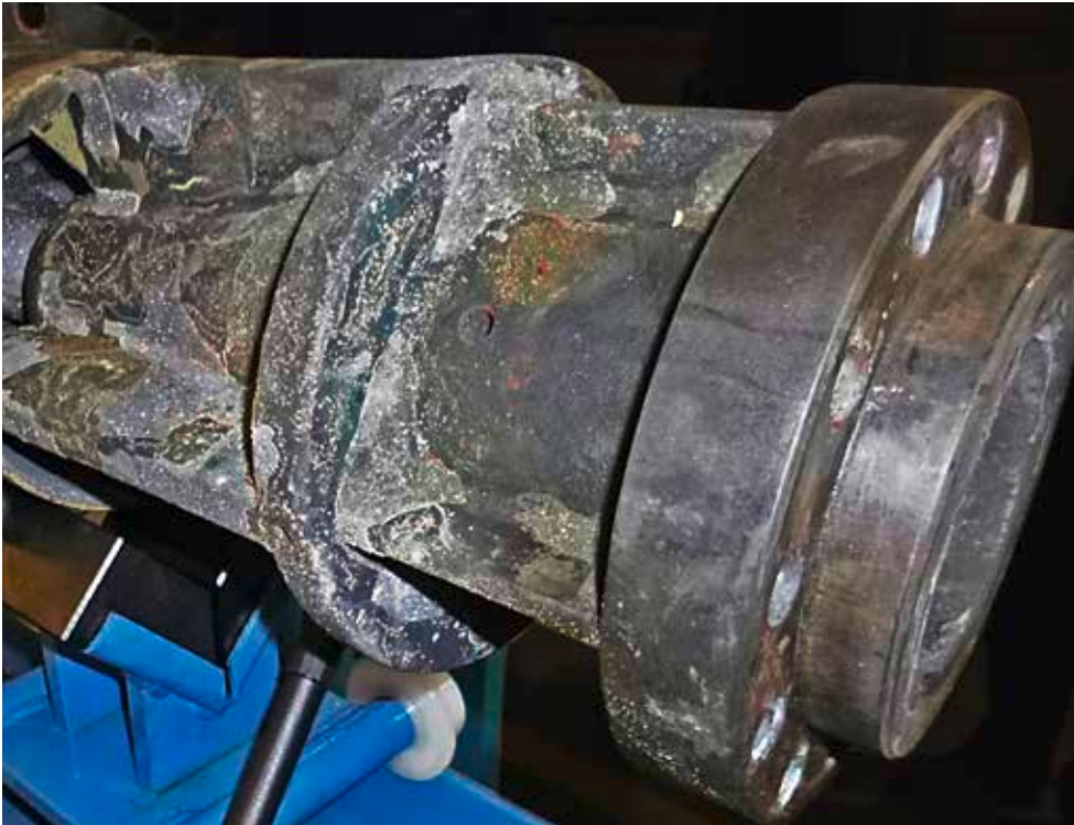
Typical limescale deposits at the pump inlet
