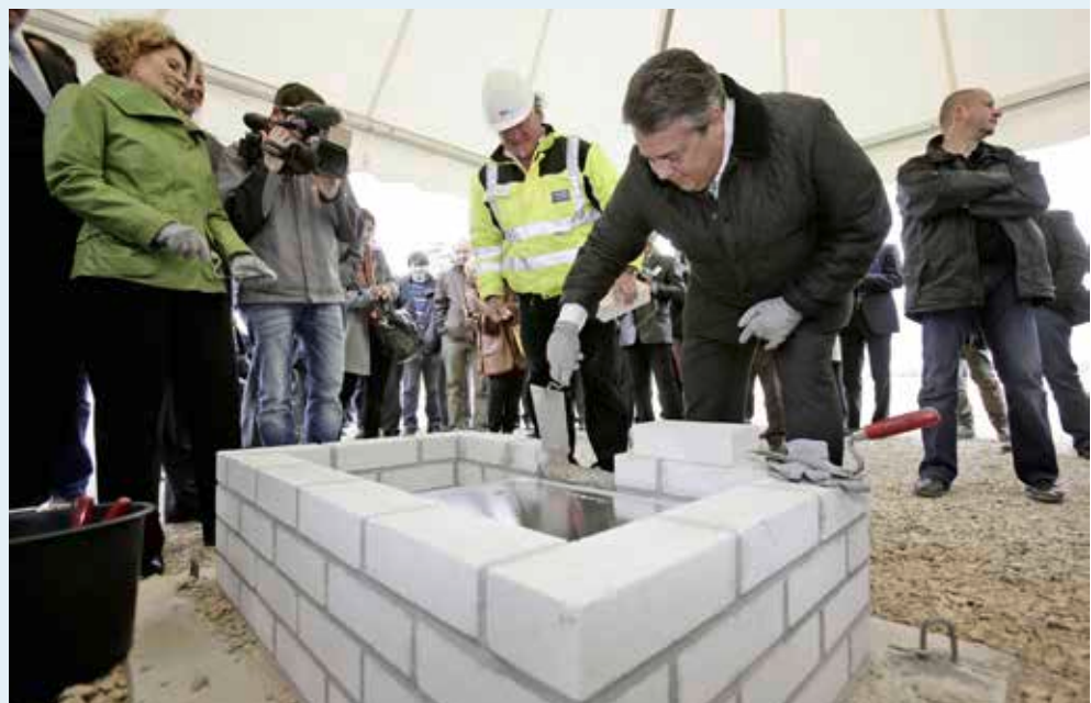
Laying of the foundation stone by the Federal Minister for Economic Affairs and Energy Sigmar Gabriel
